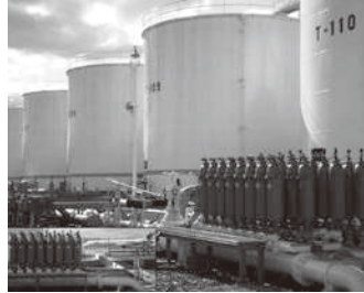
Shock dampening for fuel supply pipings to the aircraft.
