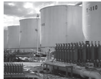
Shock dampening for fuel supply pipings to the aircraft.
